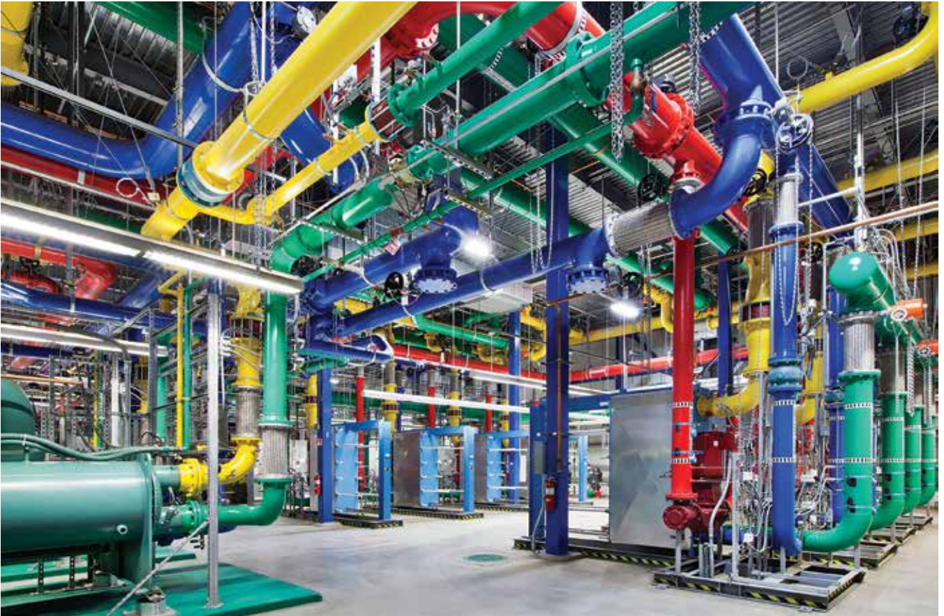
In 2005, Google sited a data center in The Dalles, Oregon, because of the city's municipal fiber network.
